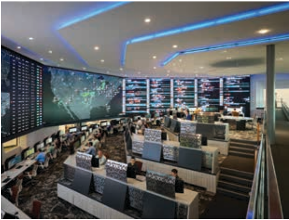
The high-tech Global Operations Control Center was inspired by NASA control centers.
